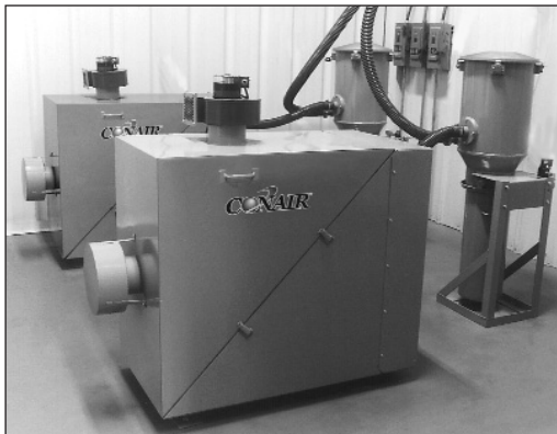
5 HP Pumps in Sound Enclosures (with dust collectors)
